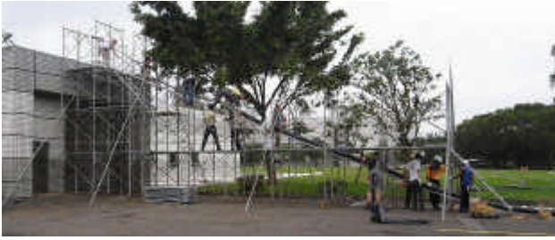
Figure 4: Scaffold to raise the flexible transfer lines from the grass yard to the TLS booster roof.
